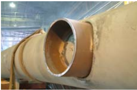
Stubs are welded into place to hold the cross ties that run between the arches.
