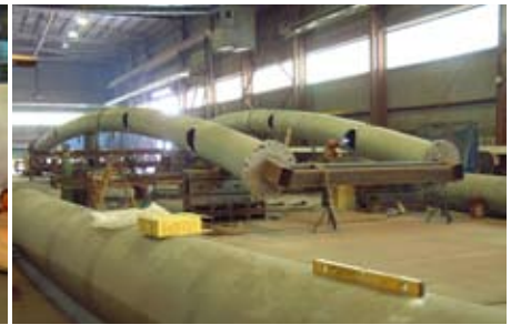
Welded and painted arch segments are trial fit one last time before shipping.
