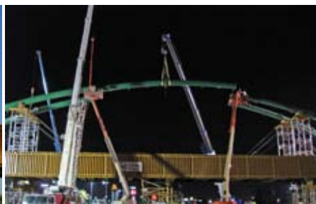
The final center section, with an arch height of 39 ft., is fitted into place.
