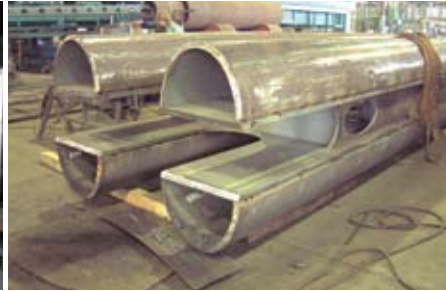
The pylon tower elliptical pieces were formed in a large press brake. Consistency in their shape was critical to making them fit together.
